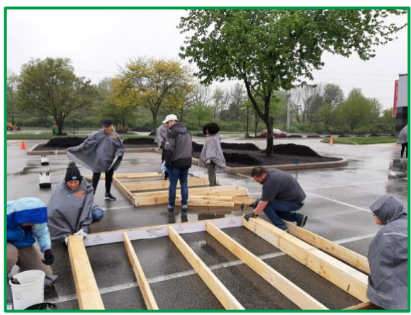
Working on wall paneling for the upcoming house on D Ave with Offprem Technologies
